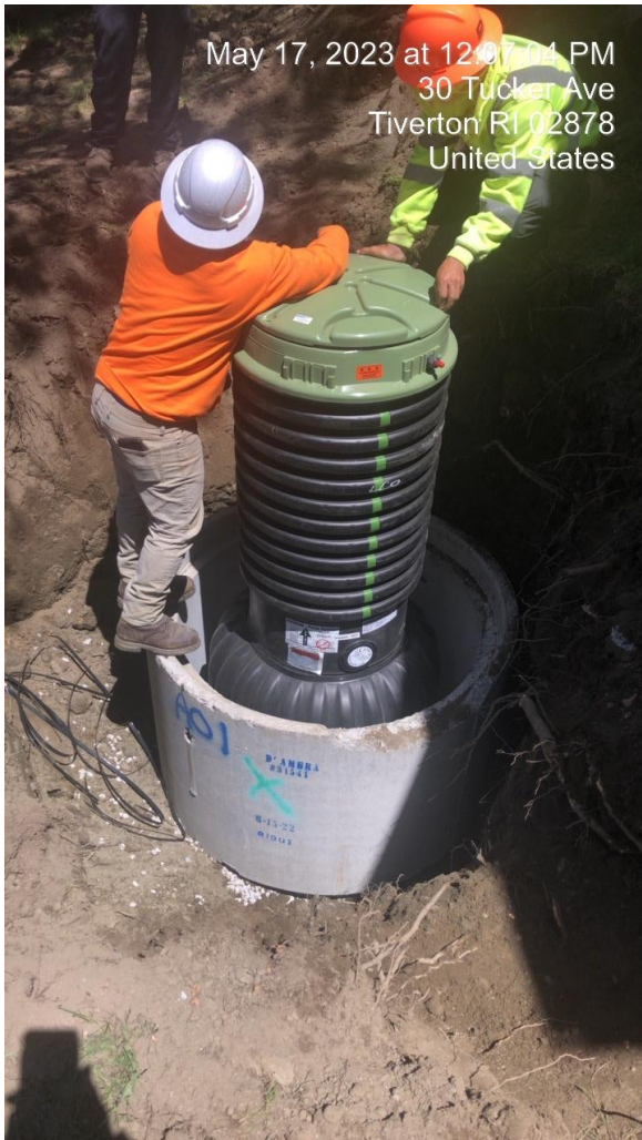
Figure 2 Grinder pump installation.
